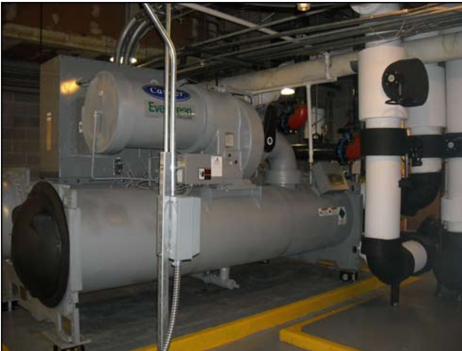
Installing the 550-ton chiller and piping required AFO to knock out a wall.
